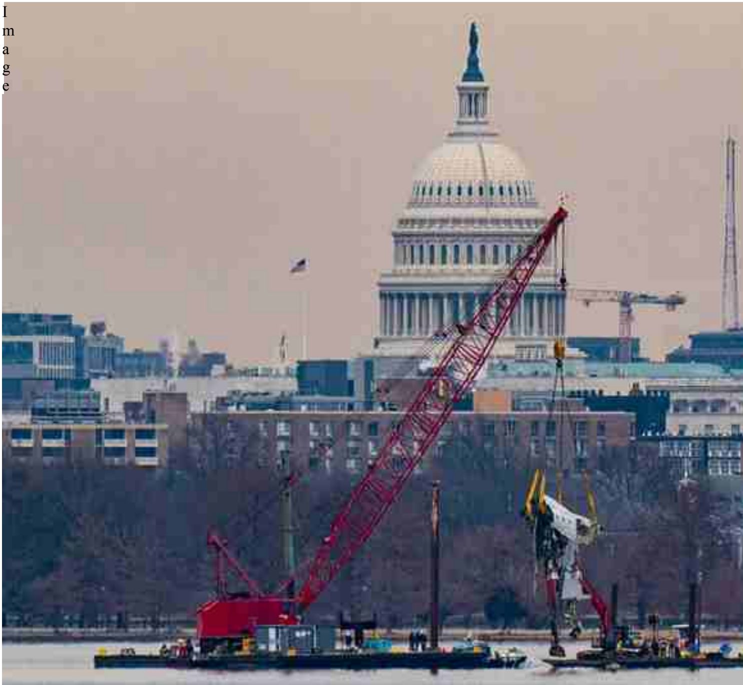
A crane removing pieces of an American Airlines plane that crashed in January from the Potomac River near Reagan National Airport in Arlington, Va. Al Drago for The New York Times
